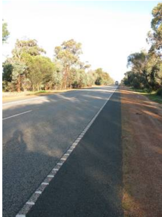
Figure 2.1 A typical treatment site with audible edge line and 1.5m sealed shoulder installed next to the 1m unsealed shoulder
